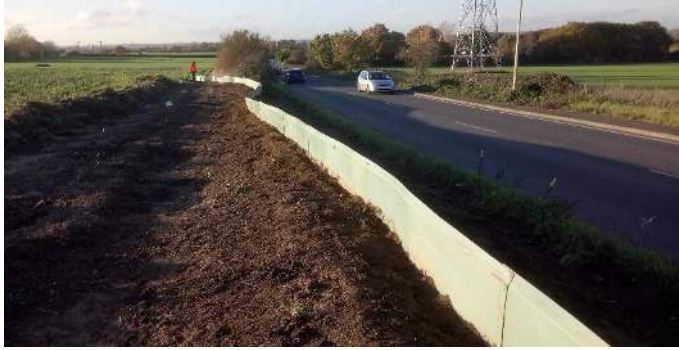
Figure 1: example image of permanent herptile fencing ('Herpetosure®' – type fencing)
